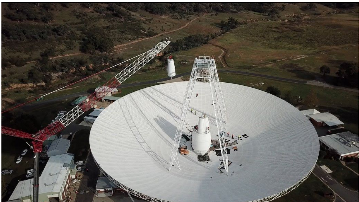
In a delicate operation, a 400-ton crane lifts the new X-band cone into the 70-meter (230-foot) Deep Space Station 43 dish located in Canberra, Australia. Image Credit: NASA/JPL-Caltech
